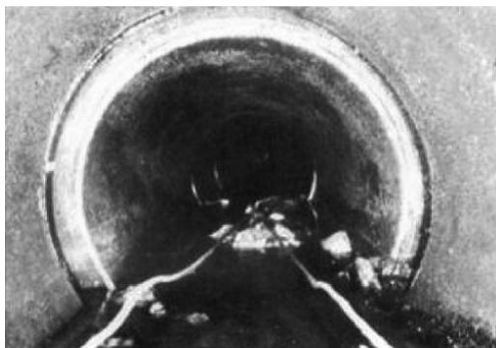
(c) 管道接口断裂
